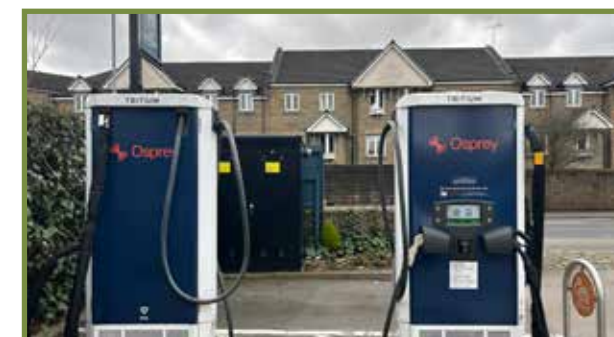
EV charging points at The Woolpack, Yeadon
